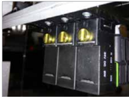
Figure 11-4 Manual override switch
