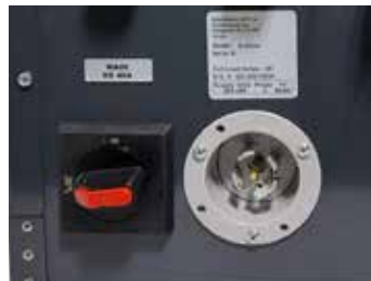
Figure 10-1 Disconnect switch and power supply connection
